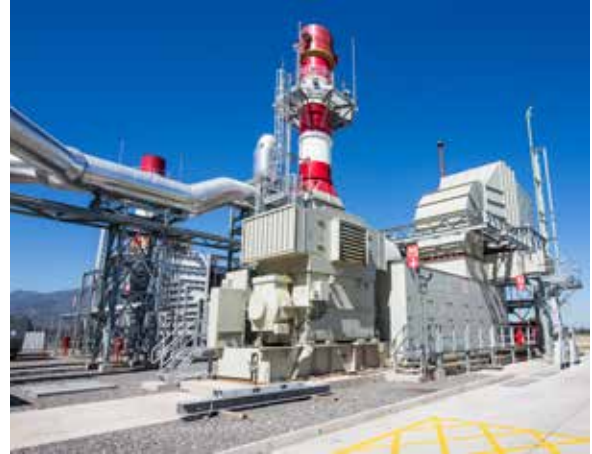
Titan 250 Generator Set - Chile
