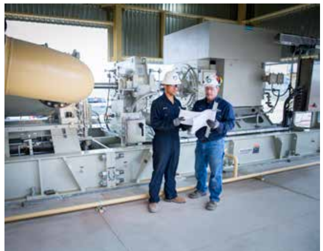
Electric Motor Drive, C33 Compressor - USA
